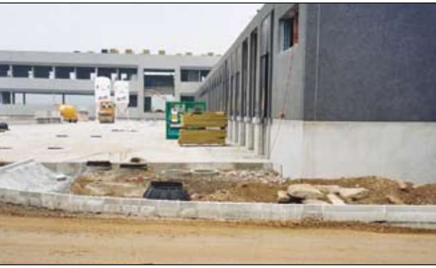
ALDI Central Warehouse: Cables for outdoor lighting
