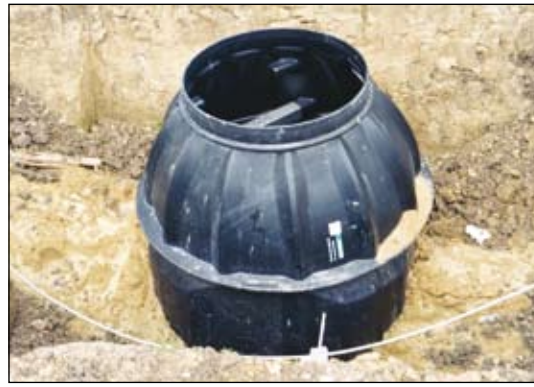
Pulling chamber with ground
